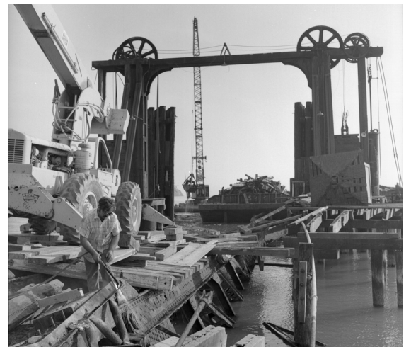
Demolition of the barge dock – Ghilotti was hired by Southern Pacific to take down the barge dock and gallows frame. Photo by Phil Molton, Feb. 1974.
