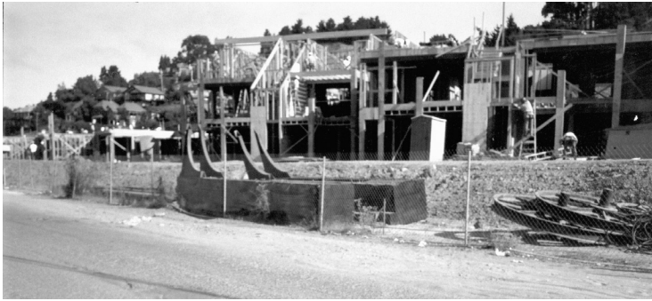
Gallows wheels and frame at Point Tiburon construction site summer 1984. (Marens collection)
