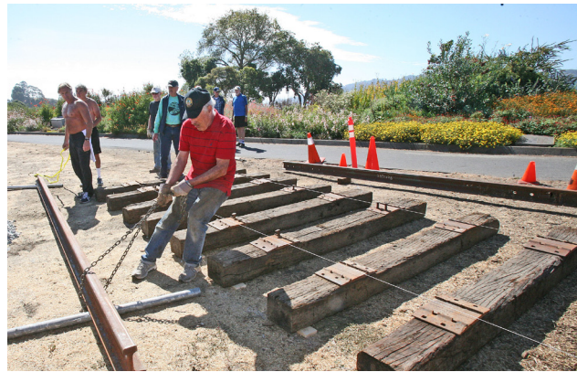
Phil Cassou, Landmarks Board Vice President and Head Docent at the Railroad & Ferry Depot Museum, heaves a 20-foot length of iron rail. Photo by Elliot Karlan.
