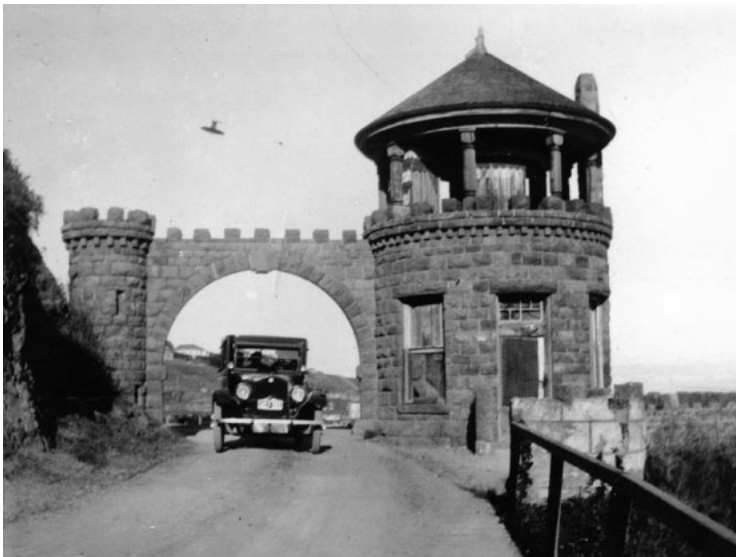
Not long before the arch was removed, this photo from the early 1920's shows the tower's condition already deteriorating.
