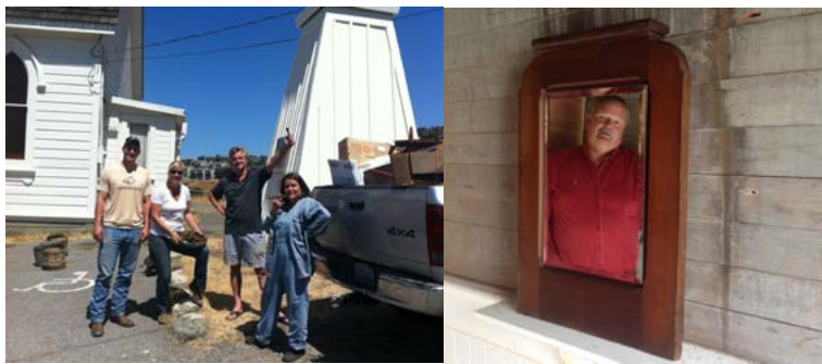
Conor & Leslie Doyle, Alan Brune, and Piper Berger clean out the old bathrooms and bell tower. Right: Mark Pearce, contractor, taking a look at how the pew door windows will fit in the new bathroom.
