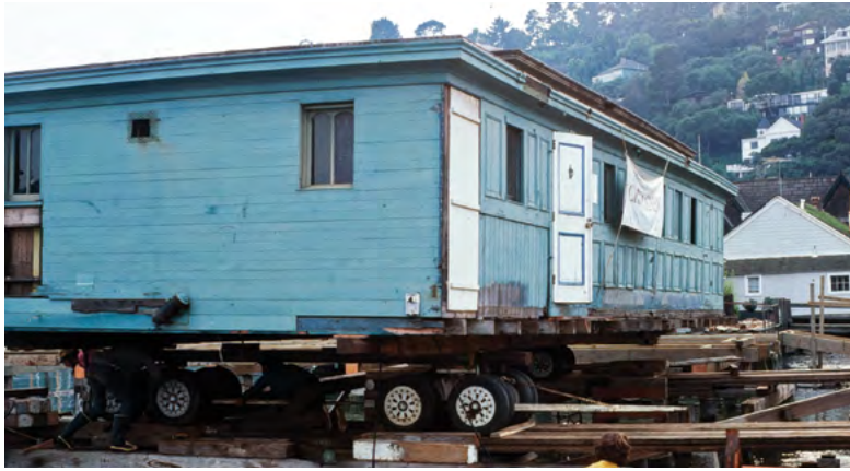
Preparing the China Cabin to be moved from its original location parallel to Beach Road to its new platform, November 1979 (George Coleman)
