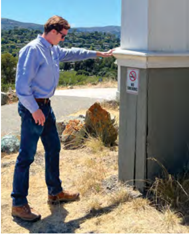
Jeff Hadley inspects the ailing buttresses at Old St. Hilary's.
